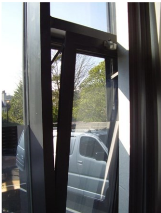
Figure 5.2 Example of ventilation area reduced by the restrictor. Column prevents window opening
